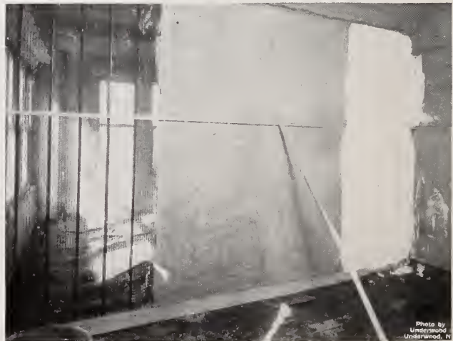
Hy-Rib Partition, without channels, E. W. Browning Apartment Hotel, New York. Showing Hy-Rib, scratch coat, second coat, and finish plaster coat. Fanning Cerra, Inc., Plastering Contractor, Buchman & Fox, Architects.
