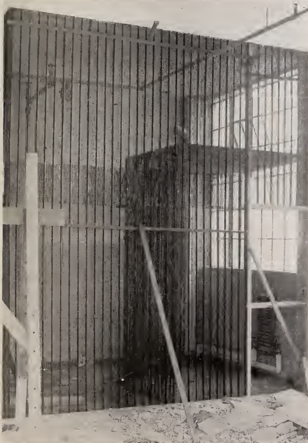
Hy-Rib partition without channels—Dodge Bros. Power Building, Detroit, Mich. Note simplicity of temporary bracing.
