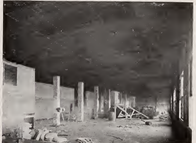
\frac{3}{8} " Hy-Rib Lath Ceiling—Hutchinson High School, Buffalo, N. Y. H. Osgood Holland, Architect; James G. Davis, Plastering and Lathing Contractors.
