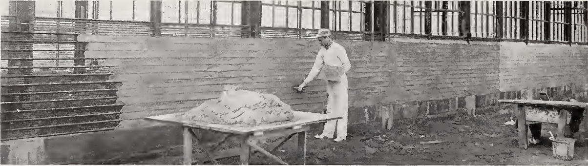
Hy-Rib Stucco Siding showing method of plastering. Note Truscon Steel Windows above.
