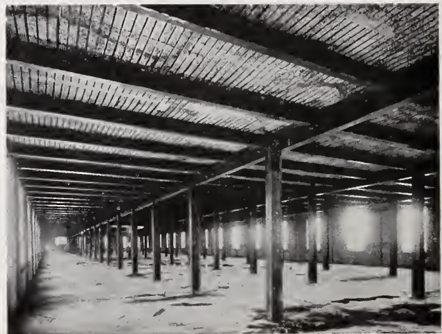
Under side of Hy-Rib floor before plastering. Edward Ford Plate Glass Co., Rossford, Ohio. De Vore-McGormley Co., Engineers.
