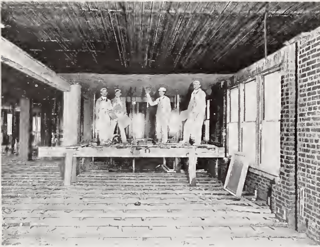
\frac{3}{8} " Hy-Rib Lath ceilings, joists 24" center to center. Kennedy Bros. Apartments, Washington, D. C. R. W. Allen, Lathing Contractor. Murray Bros., Plastering Contractors.
