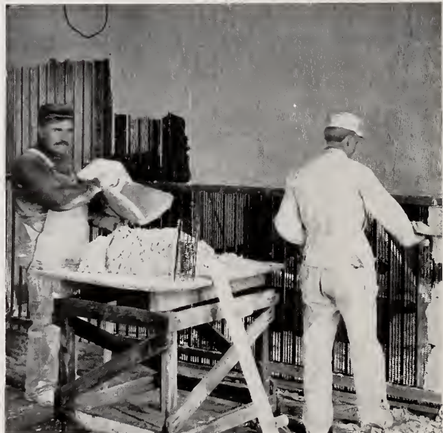
Solid Partitions without Channels. Ribs of Hy-Rib extend from Floor to Ceiling. Owen Building, Detroit.
