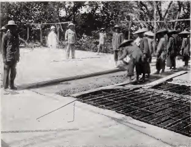
Pouring concrete floor, reinforced with 1½" Hy-Rib. St. Andrew School, Singapore, Straits Settlements. Note Chinese women carrying concrete in buckets.
