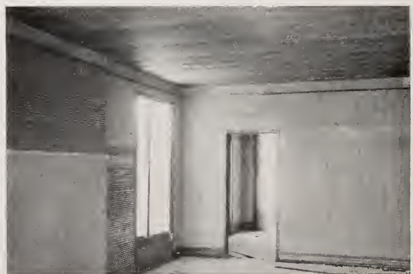
Hy-Rib Lath for Walls, Partitions and Ceilings. Residence of J. B. Book, Jr., Detroit, Mich.
