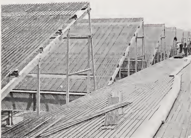
Hy-Rib Saw-tooth Roofs before concreting., Oliver Chilled Plow Co., Hamilton, Ont. David Dick & Son, Contractors. Prack & Perrine, Architects.
