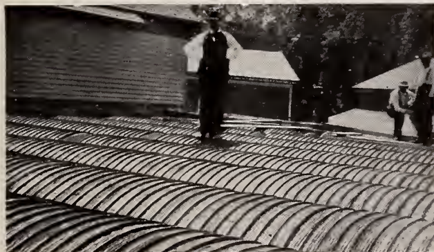
Arched Hy-Rib Floor in Joseph Bendt Store, Kenosha, Wis., used in conjunction with reinforced concrete beams.
