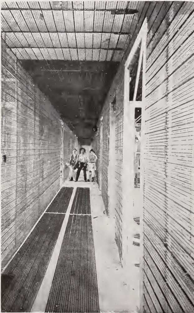
Hy-Rib Lath throughout interior for partitions and ceilings. Plaza Hotel, Dallas, Texas. Guidera & Bell, Owners, Architects and Contractors.
