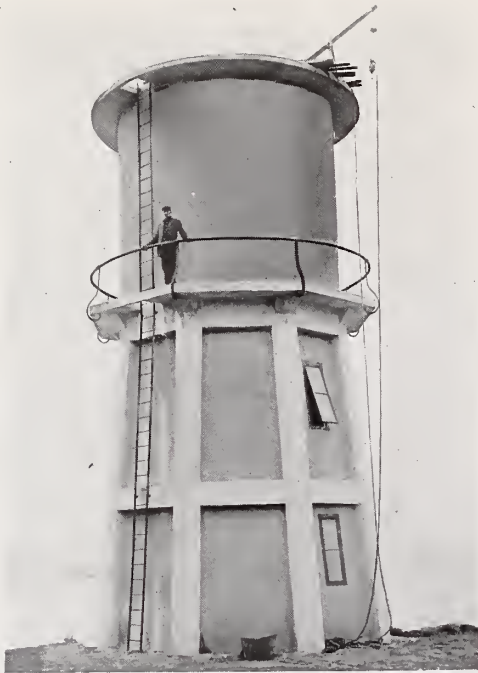
20,000-Gallon Tank, Marine Biological Station, San Diego, Cal. Irving J. Gill, Architect. Tanks and Panels are Hy-Rib Concrete. Posts and Girders are Truscon Reinforced Concrete.
