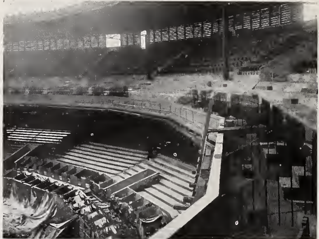
National League Baseball Grandstand, Cincinnati, O. Hy-Rib Concrete Partition Walls around boxes, etc.
