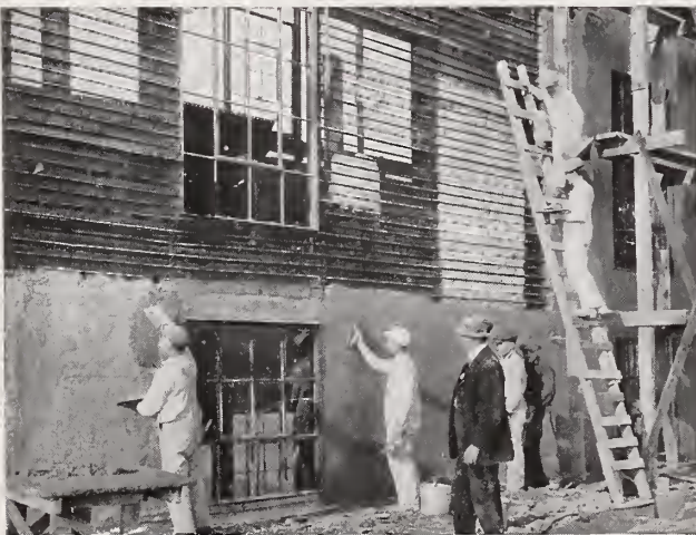
Hy-Rib Sidings of Grain Elevator, Husted Milling Co., Buffalo, N. Y. A. E. Baxter & Co., Consulting Engineers. Monarch Engineering Co., Contractors. James G. Davis, Plastering Contractor.
