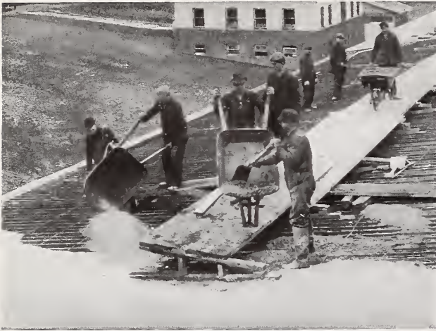
Concreting 1½" Hy-Rib on roof of a building at our Youngstown Plant.
