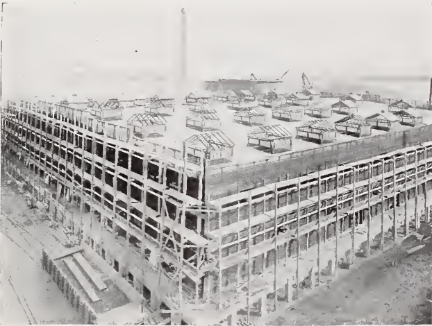
U. S. Bonded Warehouse, Curtis Bay Distillery. Hy-Rib applied to side walls ready for plastering.
