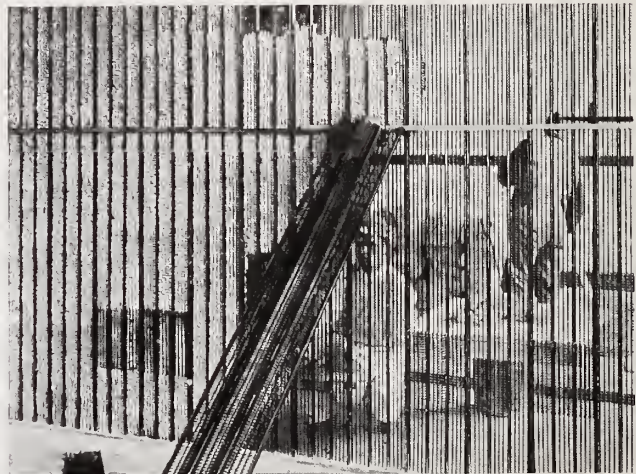
Plastering Hy-Rib Partition as viewed from opposite side. Note perfect clinch with no drooping of plaster.
