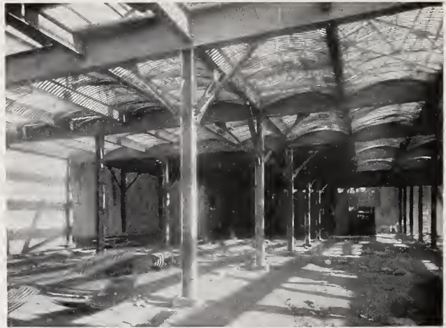
Arched Hy-Rib floors, Hawaiian Pineapple Co., Honolulu, T. H. View from below showing Hy-Rib ready for concreting. Clear spans of 7' 6" without use of forms or supports.
