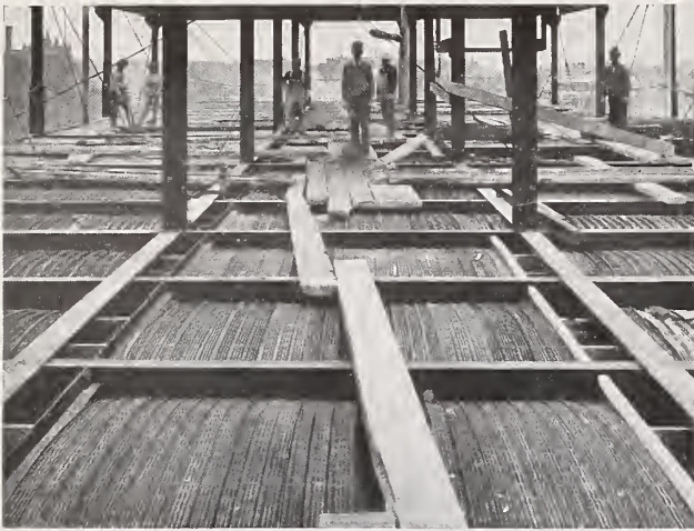
St. Mary's Hospital, Milwaukee, Wis. Esenwein & Johnson, Archts. J. D. Gregg, Supervising Archt. Arched Hy-Rib floors throughout. Hy-Rib ready for concreting.
