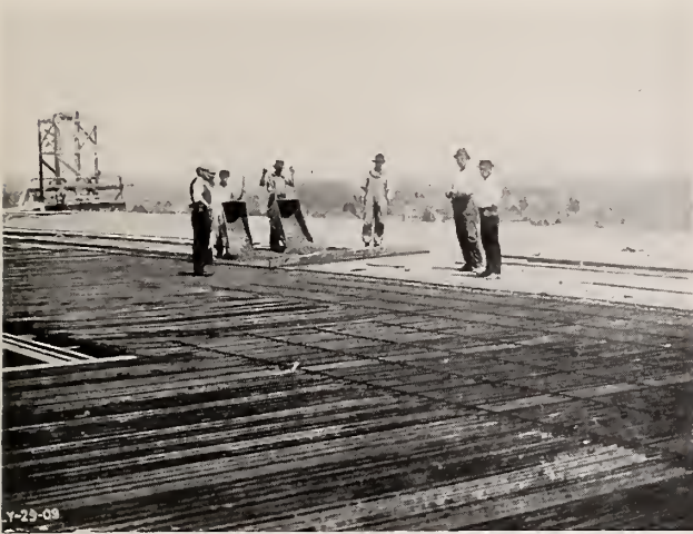
Hy-Rib Roof for Packard Motor Car Co., Detroit, Mich. Albert Kahn, Architect. Ernest Wilby, Associate.
