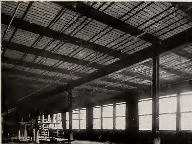
\frac{3}{8} " Hy-Rib Lath on Channels, 30" centers. Crown Building, Cleveland. Forest City Engineering Co., Architects and Engineers. Masters & Mullen Company, General Contractors.
