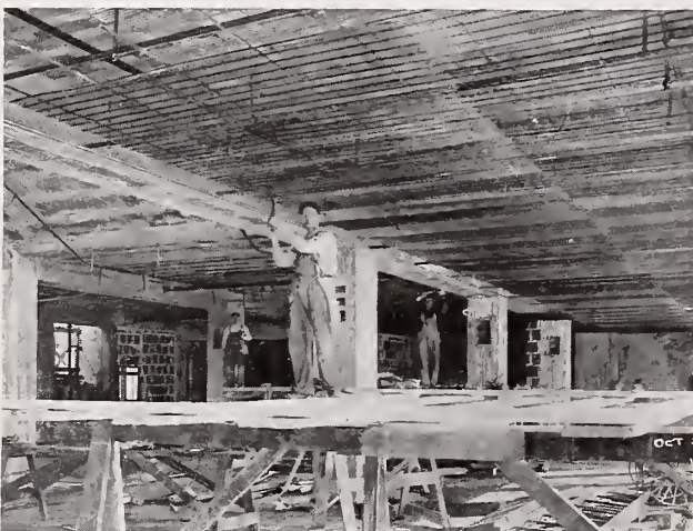
Hy-Rib suspended ceiling, B. J. Johnson Soap Co., Milwaukee, Wis. Lockwood, Greene & Co., Architects and Engineers.
