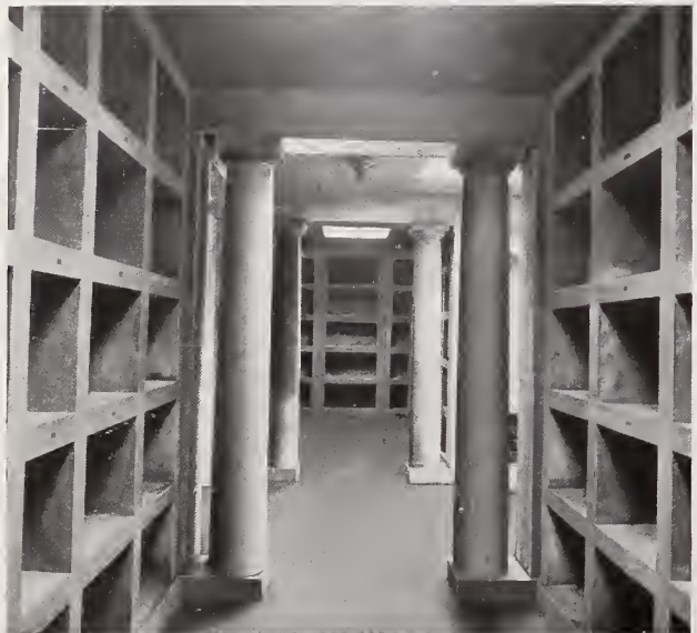
Mausoleum, Detroit Crematorium, Detroit, Mich. Partitions, niches, columns and beams are Hy-Rib Concrete.
