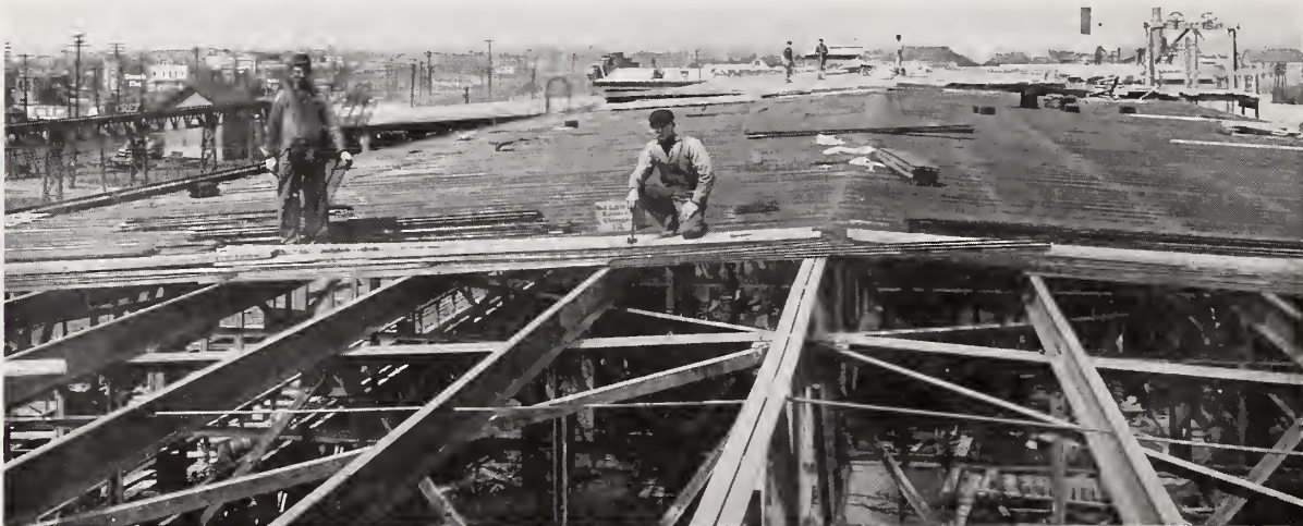
Hy-Rib Roofs, Featherstone Foundry, Chicago, Ill. Note Steel Purlins ready for Hy-Rib Sheets, and Hy-Rib ready for Concrete.
