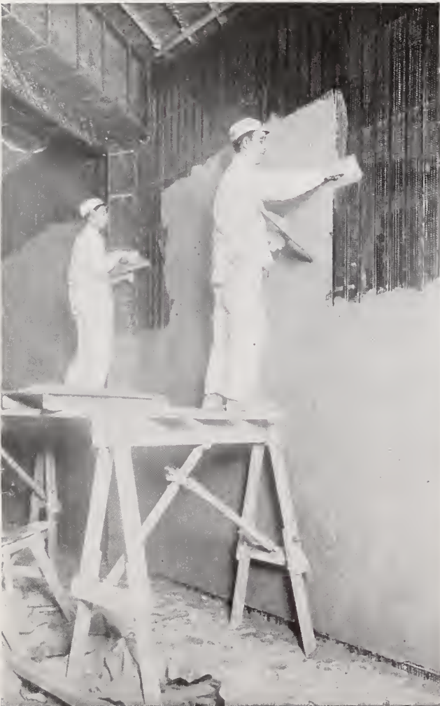
Hy-Rib Partitions, 15 feet high, Merchant's Realty Co., Detroit, Mich. Note extreme height without use of studs or supports, also heavy first coat of plaster made possible by key and stiffness of Hy-Rib.
