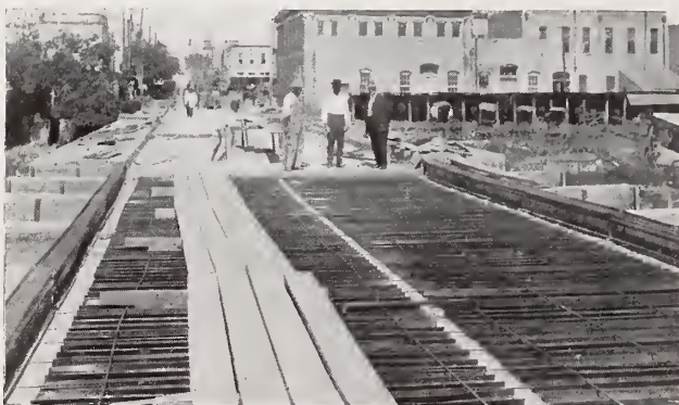
Concrete Bridge Floor reinforced with 1 1/2" Hy-Rib—Viaduct over Nolan Creek, Belton, Texas. Hy-Rib in foreground ready for concreting; floor in background completed.
