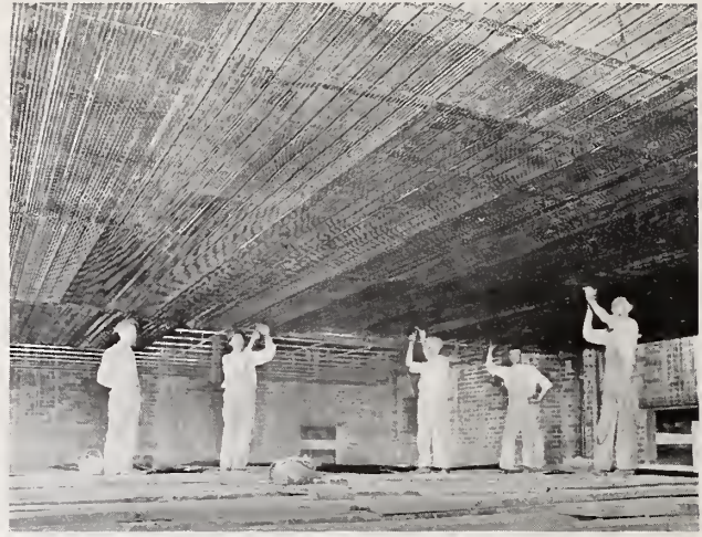
\frac{3}{8} " Hy-Rib ceiling supported by Pressed Steel Channels. Miller School, Akron, Ohio. Indiana Engineering & Construction Co., Contractors. Neirmaier Bros., Lathing Contractors.
