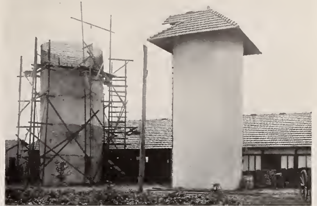
Hy-Rib Concrete Silos for J. R. Cross Co., Jersey Farms, Fairhope, Ala.
